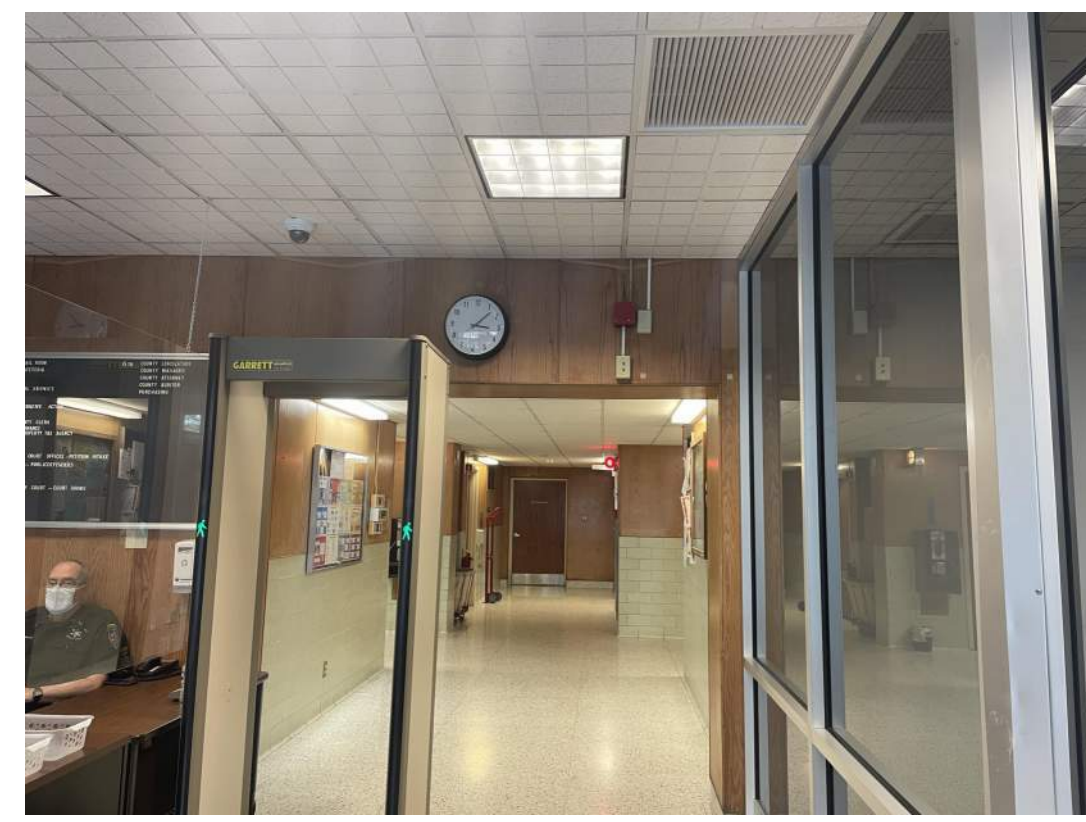
2. EXISTING FIRE ALARM BOX, WALL MOUNTED CLOCK, SECURITY DETECTOR, AND REMOVAL OF WOOD PANELING
